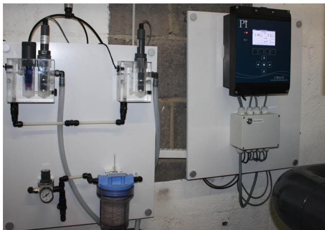
Fig.3 - A picture of one of the CRIUS® controllers installed at Crow Wood Leisure.
